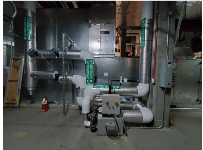
Key Hall AHU 14:
