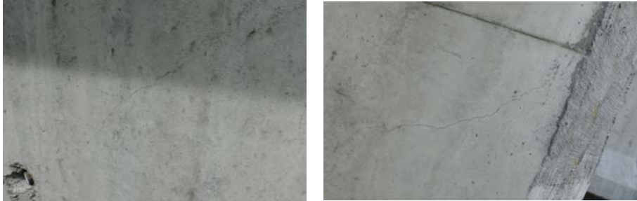
Figure 7: Beam end cracks of prestressed concrete I-beams stored at NPP
