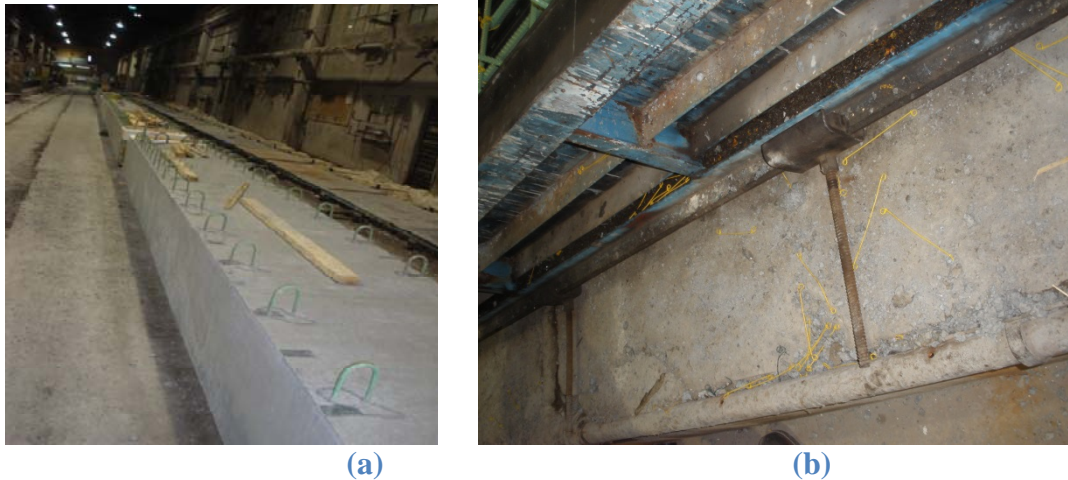
Figure 9: Finished prestressed beams with some (a) hairline cracks and (b) spalling
