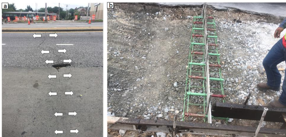
Figure 18. Subgrade differential settlement, (a) continuous surface crack on asphalt pavement and concrete bus pad, (b) poor leveling of subgrade surface before concrete pouring at joints
