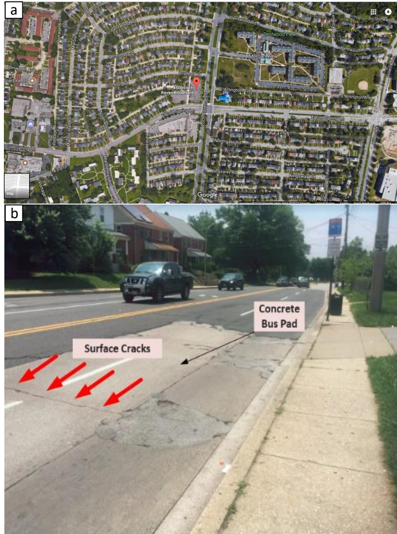
Figure 1. Field location and problem observation, (a) location of taking the field samples, (b) surface cracks were observed on concrete bus pad designed for Baltimore City
